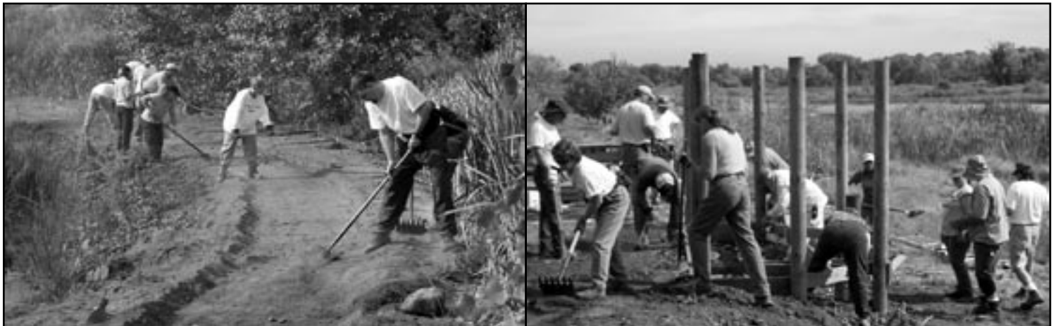
Photos left: VOC volunteers work to get the trail surface prepared for the crusher fine gravels. Right: Volunteers begin constructing the bird viewing blind and creating the trail that leads visitors into the blind. Photos by Kent Wiley, ASGD board member.
